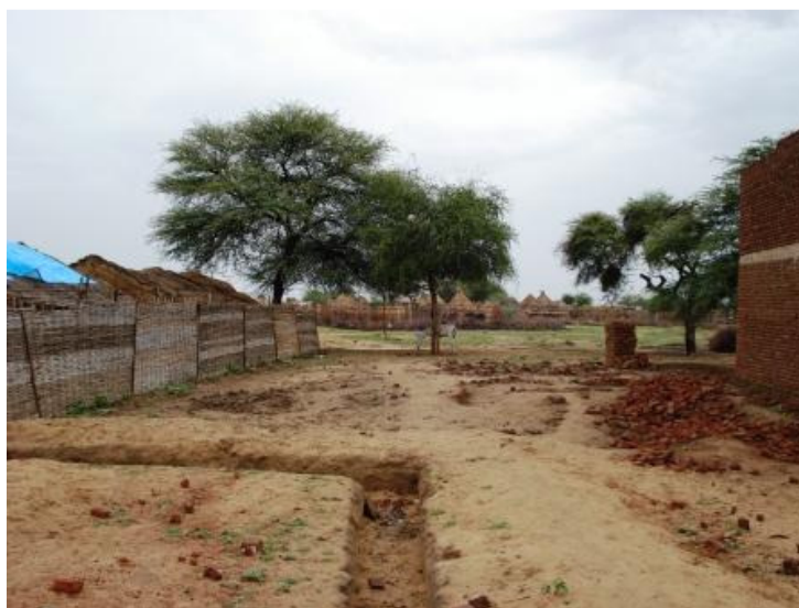
Dreeb Alrih area in South Darfur, a construction site of one of the ZOA projects.
